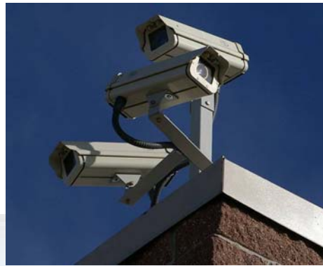
Figure 1: A CCTV surveillance system makes use of a video camera imaging system that transmits a signal to a specific place, on a limited set of monitors.
